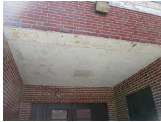
Worn Soffit Paint
