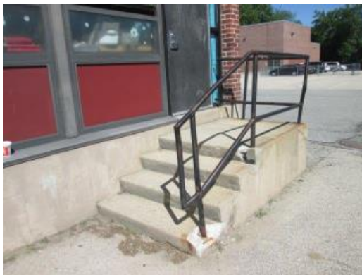
Damaged Exterior Stair Railing
