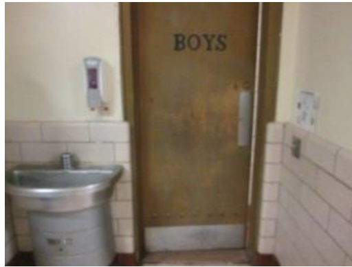
Worn Interior Wood Door
