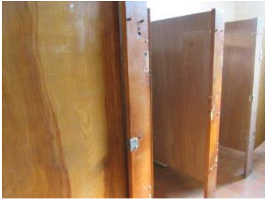
Damaged Toilet Partitions
