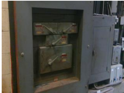
Main Distribution Panel
