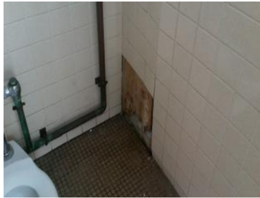
Damaged Tile Wall In Boys Restroom
