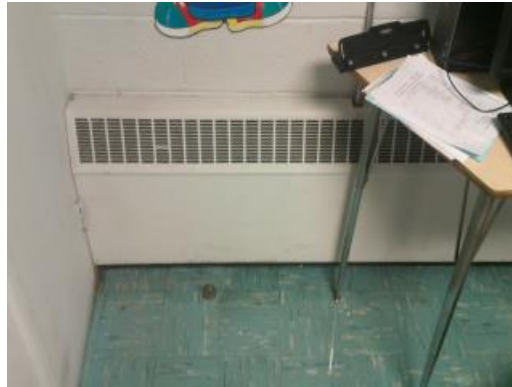
Hot Water Radiator
