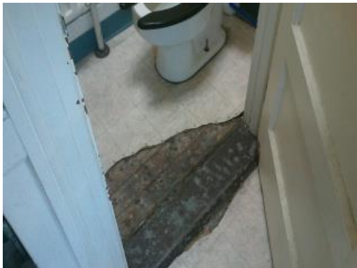
VCT Tile Damage In Faculty Restroom
