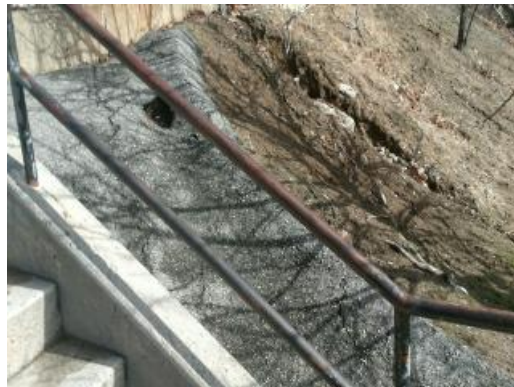
Rusted & Worn Stairwell Railing
