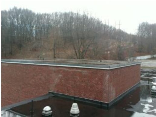
Roof Ponding - Gym Area
