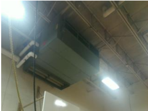
Make Up Air Unit
