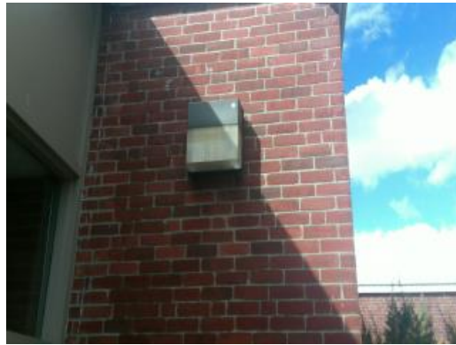
Building Mounted Light
