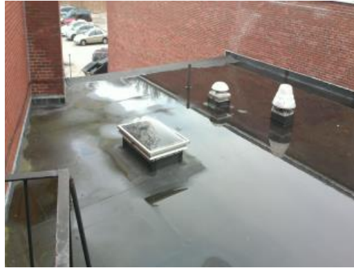
Ponding On Roof
