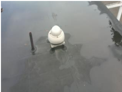
Small Roof Exhaust And Roof Ponding
