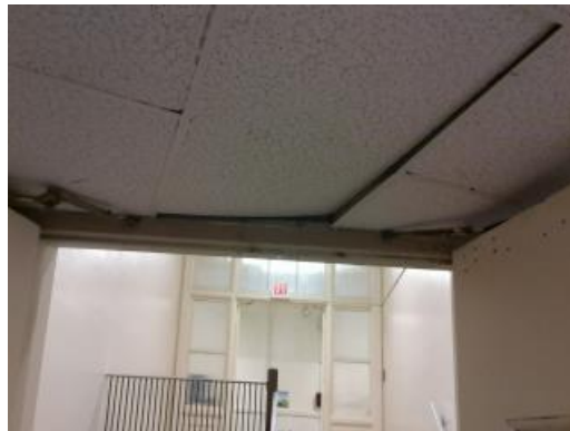
Ceiling Grid And Tiles
