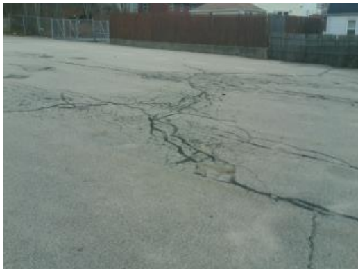
Cracked Asphalt Paving
