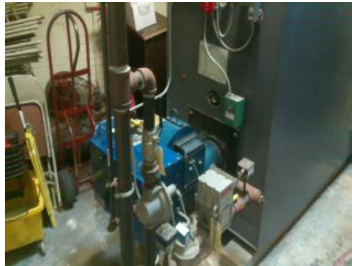
Hot Water Boiler
