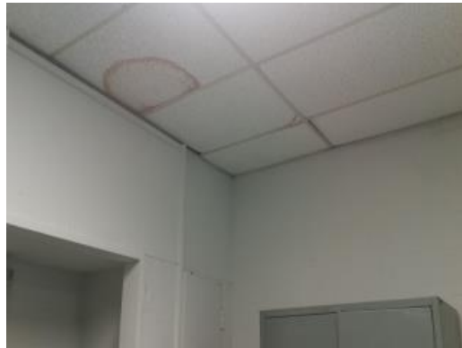
Stained Ceiling Tile
